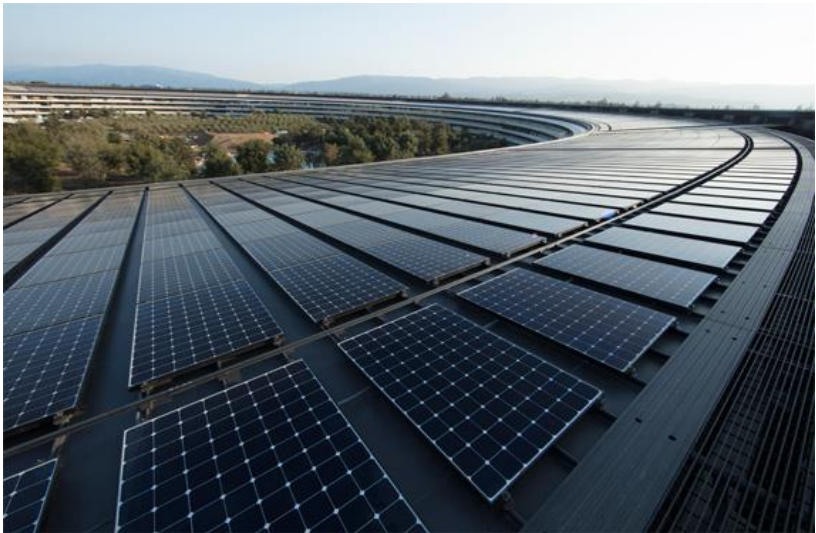
Figure 4 – Apple’s 17-MW solar installation at the new headquarters in Cupertino, California (United States). This solar installation could generate enough power to supply the entire facility (Apple, 2018).
