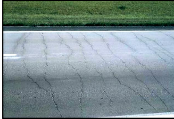
Figure 2.5 - Transverse Cracking field example (National Cooperative Highway Research Program 1997)
