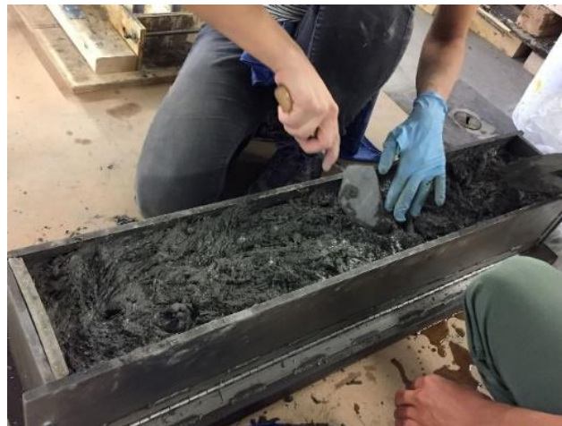
Figure 4-26 Roughening of the surface of beam IE1C2
