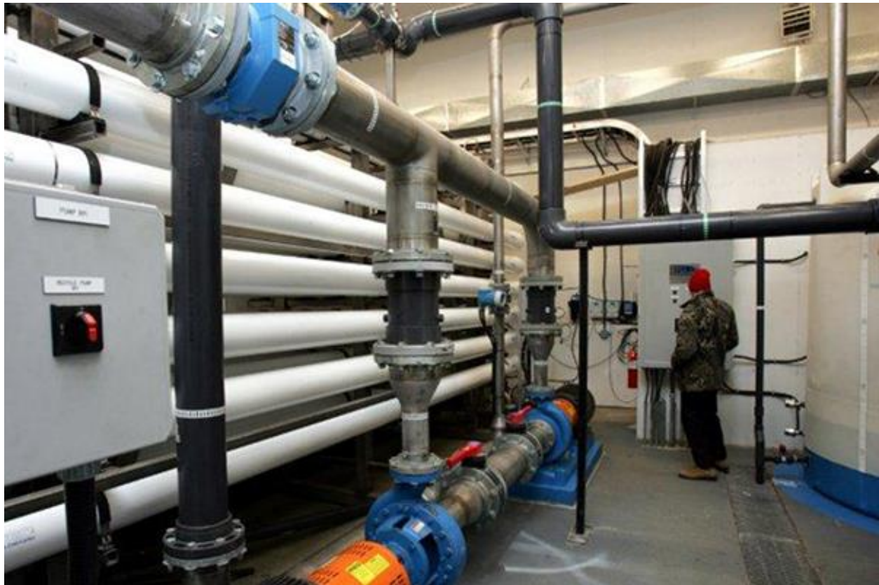
Figure 16. Inside a water treatment plant. Source: INAC, Maintenance Management Plan for Drinking Water and Wastewater in First Nations Communities, 2014.
