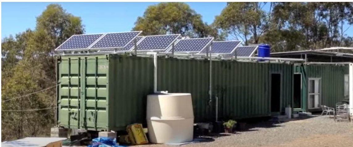
Figure 35: Solar-container system: Australia
