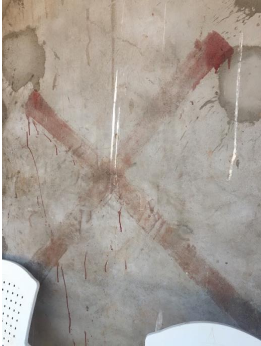
Figure X: X Marks the Spot – Due to the need to expand the access road to the Mkuju River Project, many homes, businesses and structures built along the road have been marked for destruction by TANROADS, the government authority for road infrastructure. As one informant told me, villagers were encouraged to build along the roads under villagization, but now those, and many others who have built over the decades, face the likelihood of their home being demolished so that the mining project can proceed. There is much uncertainty around compensation for the homes, mainly who will pay it and who will receive it, and many of these structures have been marked for multiple years, some since 2012. Because of this uncertainty many fear the eventual removal of their properties and the limited (if any at all) compensation that they anticipate will be attached to it (Photo: author).
