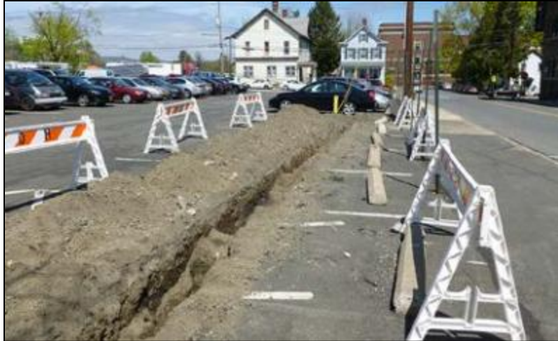
Figure 30: Expensive Trenching Required to Install Charging Station in an Existing Parking Lot (U.S. Department of Energy, 2015, p. 14)
