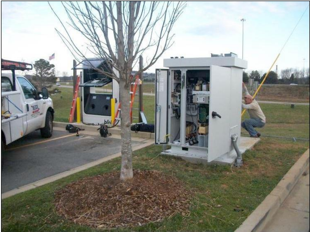
Figure 27: Installation of a costly DC Fast Charging Station (ECOtality North America, 2014, p. 84).
