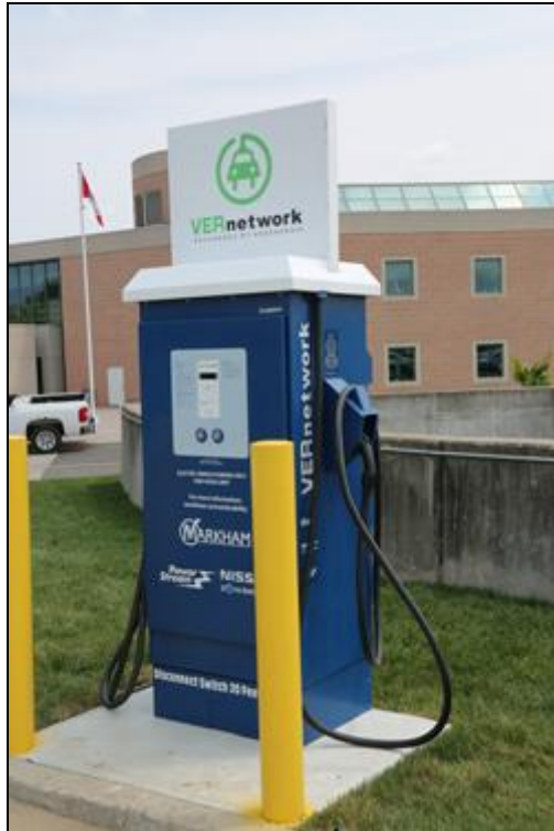
Figure 24: City of Markham's DC Fast Charger (City of Markham, 2016)
