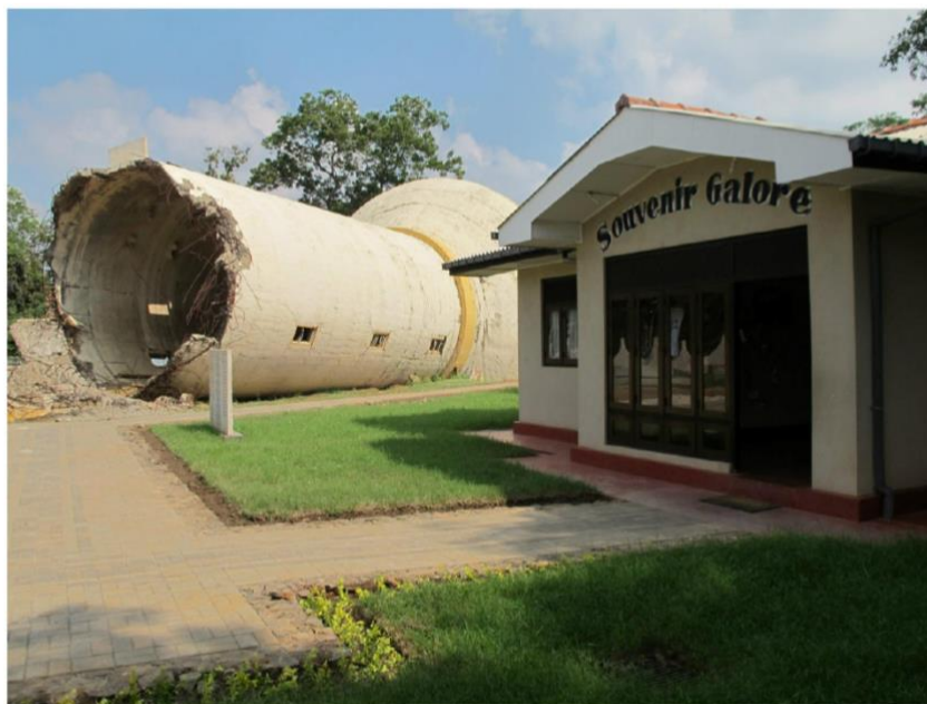
Fig. 7. Destroyed water tank in Kilinochchi with a newly built souvenir store next to it.
