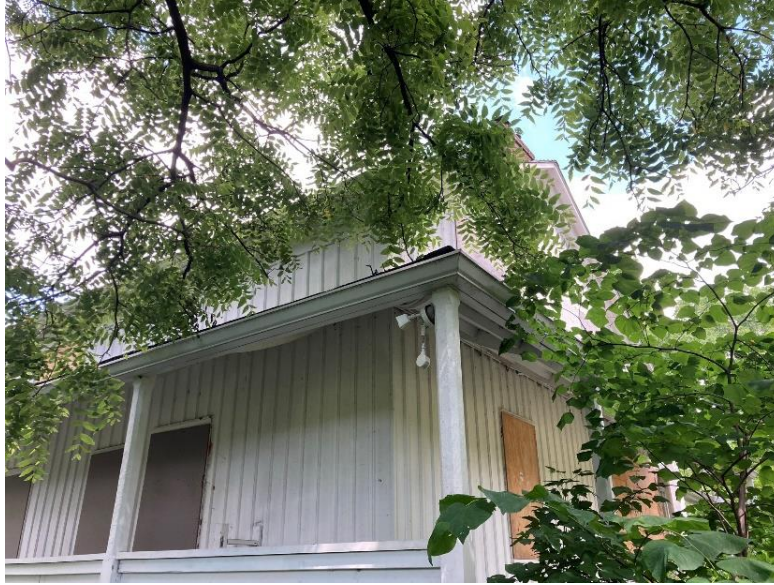
Figure 4.1: Tree adjacent to the house touching the roof (author's photo)
