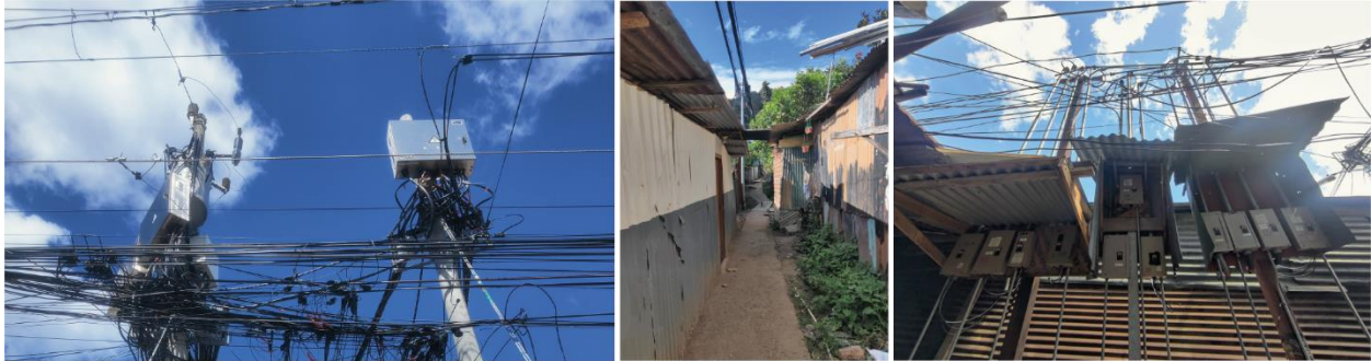
Figure G4. Grouped metering (Author's photos).
