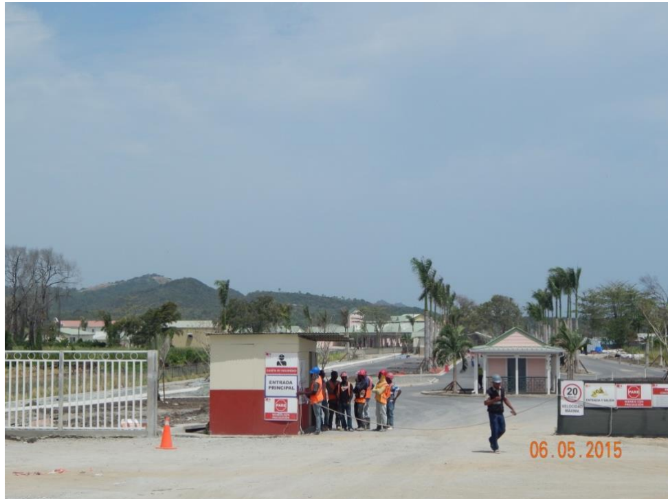
Figure 1: The early days of construction of Amber Cove Cruise Terminal. Photo by author, 2015
