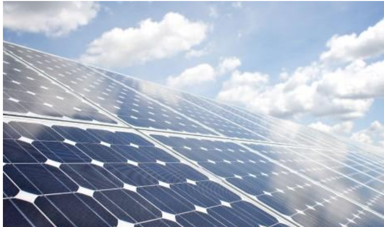
Power plant - Photovoltaic
