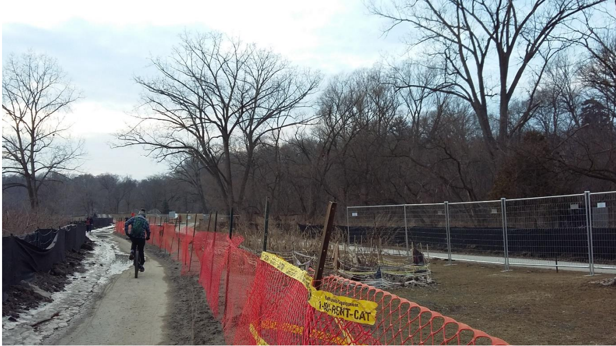
Figure 4. Etienne Brulé Park under construction with fenced in on the right the remains of last year's gardens.
