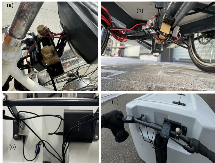
Figure 9: Device Installation on the ECCs
