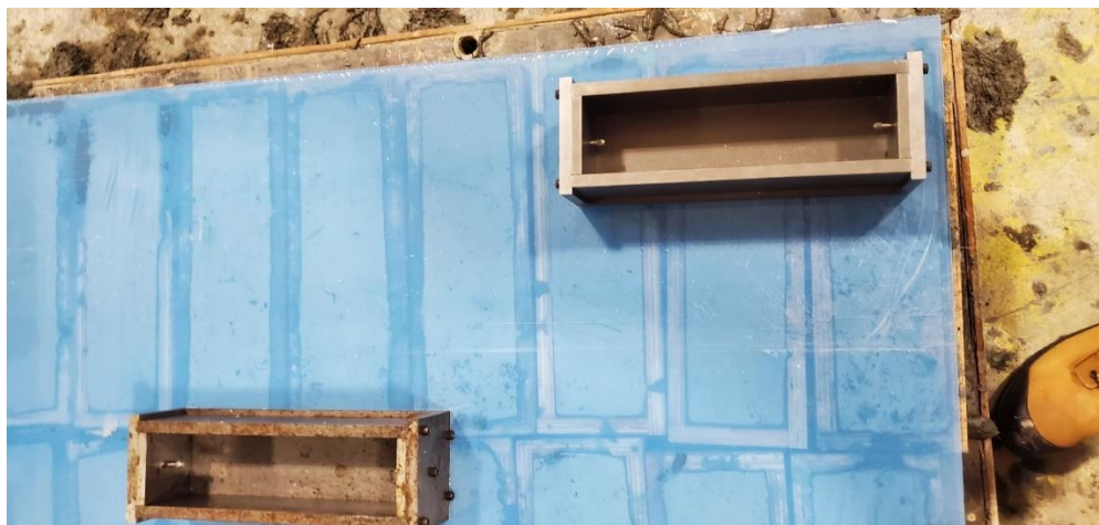
Figure 26: Flexure prism molds covered with plexiglass and empty molds to help level the finish surface.
