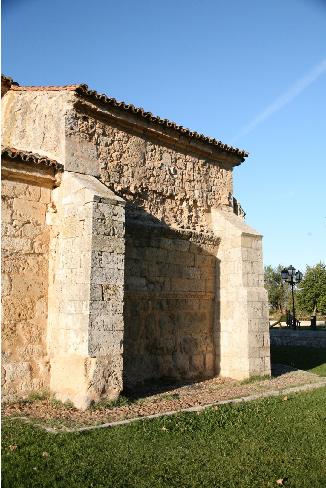
Figure 28.3: San Juan de Baños, Palencia, fragmented masonry, former barrel-vaulted south chapel.
