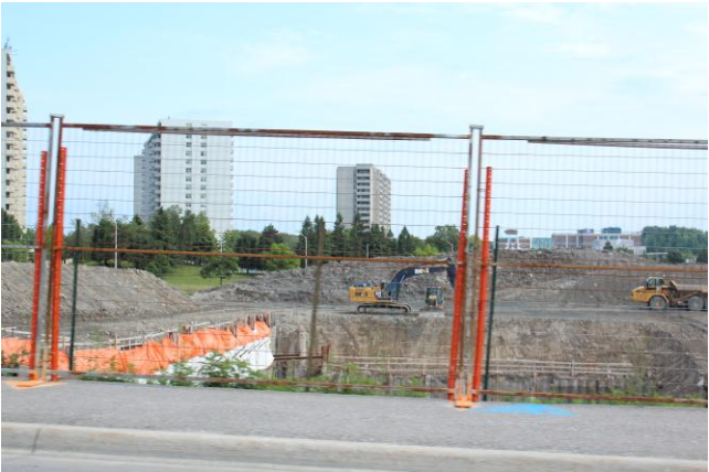
Figure 10.0 Construction underway on the southeast corner of the Harwood Ave. and Bayly St. intersection for the first phase of the downtown intensification project.
