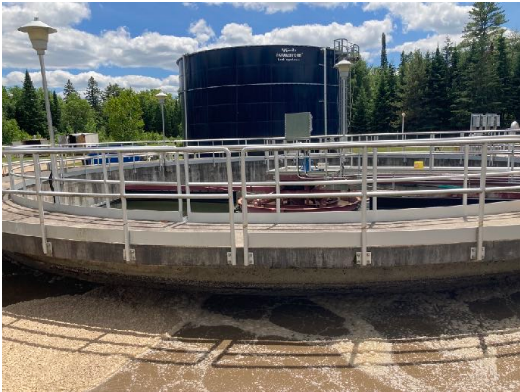
Figure 48: Bancroft Waste Water Treatment Plant (Photograph by Author)
