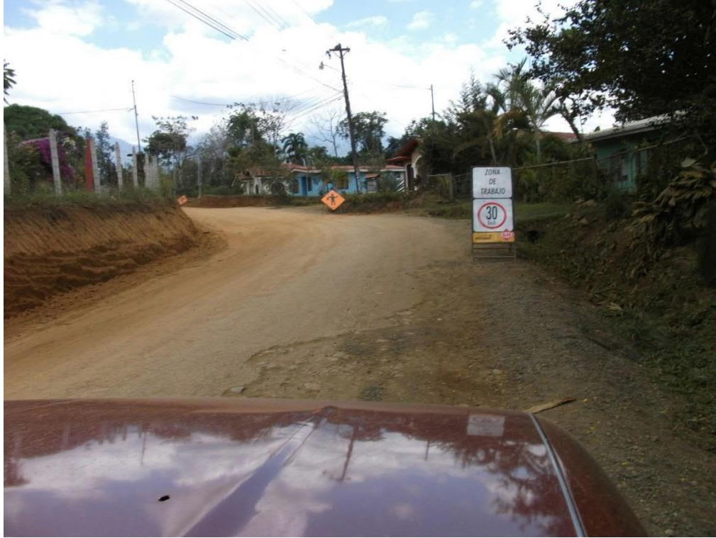
Fig. 6.3 Paving of the main road through the corridor (Alexander Skutch Biological Corridor, photo by M. Thornbush, March 2020)
