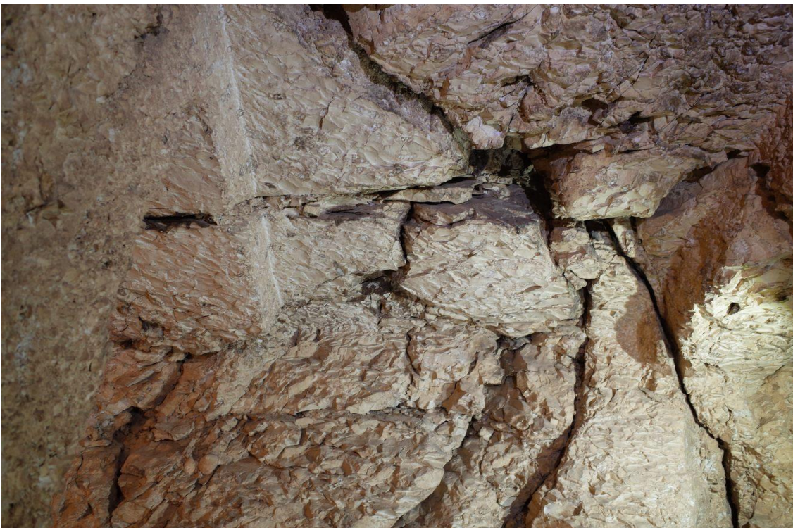
Figure 41: Exposed rock blocks suspended from the ceiling that look balanced by interlocking forces with neighboring blocks
