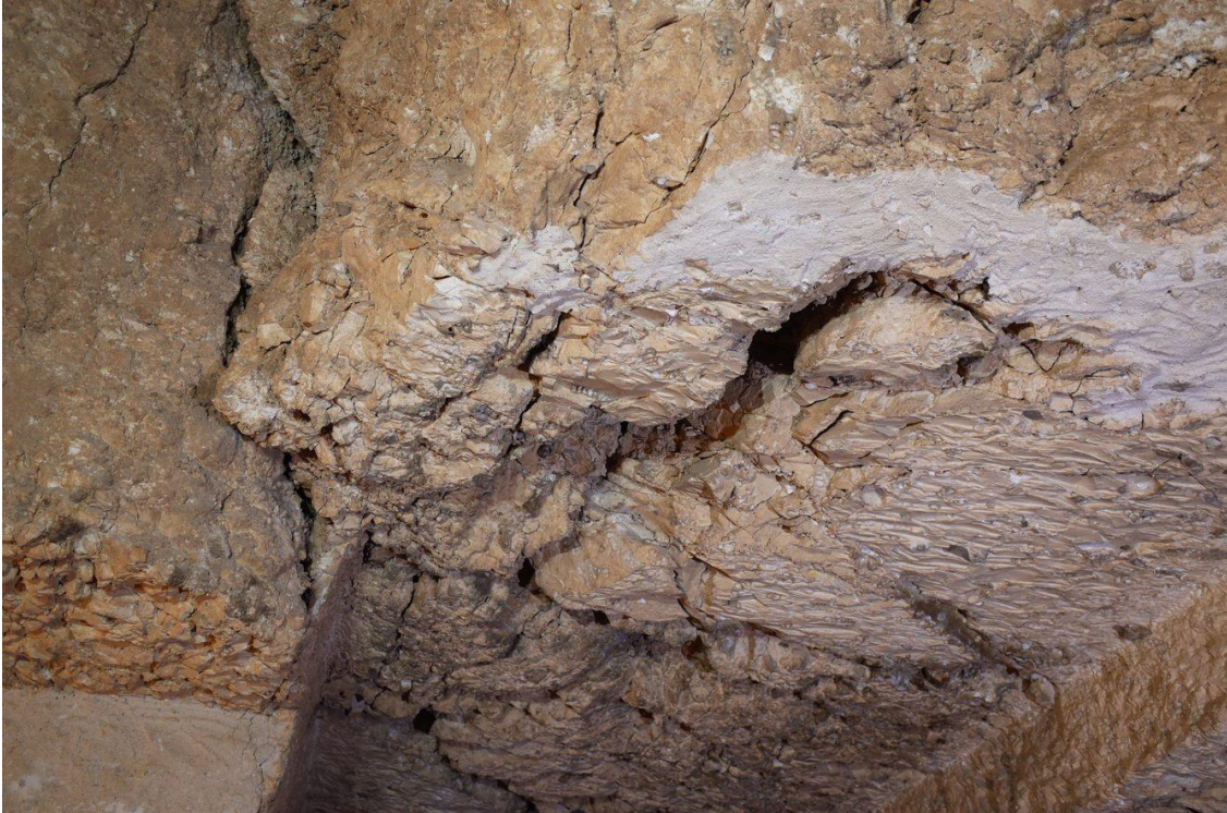
Figure 40: Fractured rock mass along on the ceiling of the South side of the main chamber
