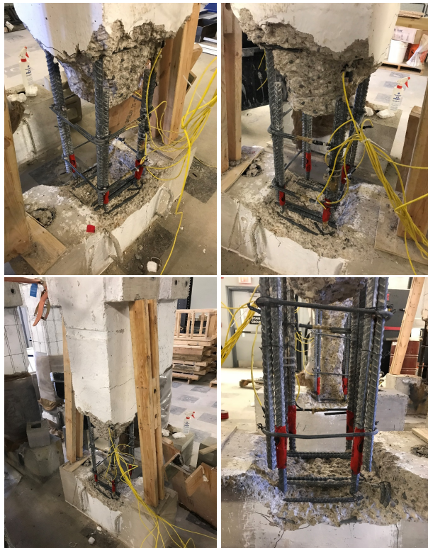
Figure C.7. Process of removal of damage cover and core concrete for specimen CT2-20M-R.
