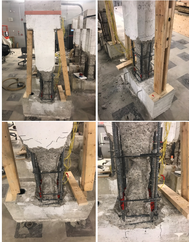
Figure C.6. Process of removal of damage cover and core concrete for specimen CT1-15M-R.
