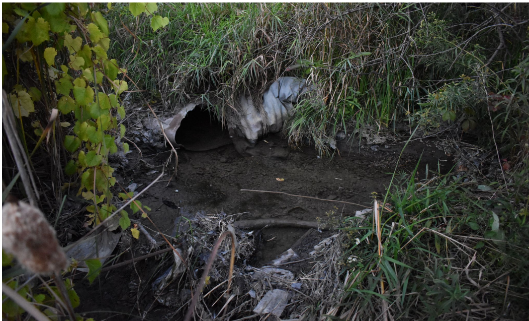
FIGURE 3-9: SITE OBSERVATIONS OF AN ERODED VEGETATED AREA ALONG THE PERIPHERY OF THE OIL TANK FARM. SOURCE: ORIANA NANO, 2021.
