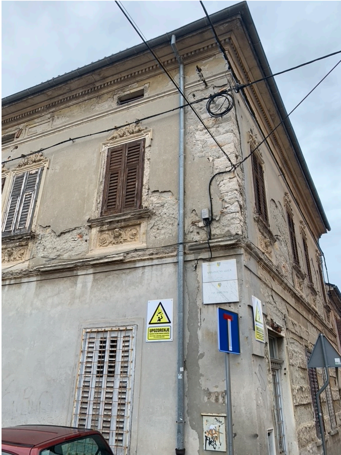
Figure 3-1. A building close to Pula's city centre. Though the home maintains some of its earlier architectural features, such as the shutters and molding around the roof and windows, much of the home's stucco facade has fallen off, revealing the structural bricks underneath. The building features a warning sign to pedestrians to watch out for falling pieces.
