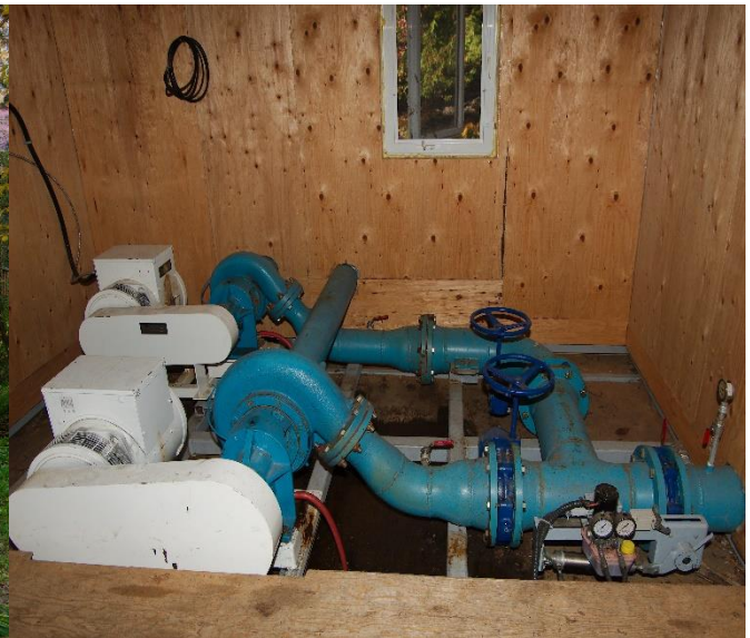
Figure 26: The Eco-Lodge's water turbine system
