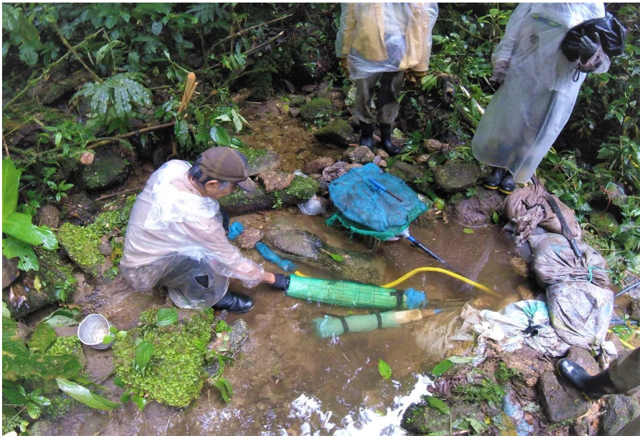
Figure 10: Yujo and the crew doing the bi-annual clean/ reset of their gravity-based water system. Sunken plastic canisters wrapped in mesh feed into hundreds of meters of pipe that snake down the mountain to the Eco Sitio. They do not filter or treat the water, and it has been functional for decades.
