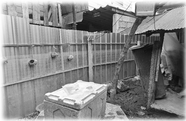
Photo 1: Traces of flood levels can be observed from the soil stains on the wall in Mae Kha community area. (Photo from the research site)
