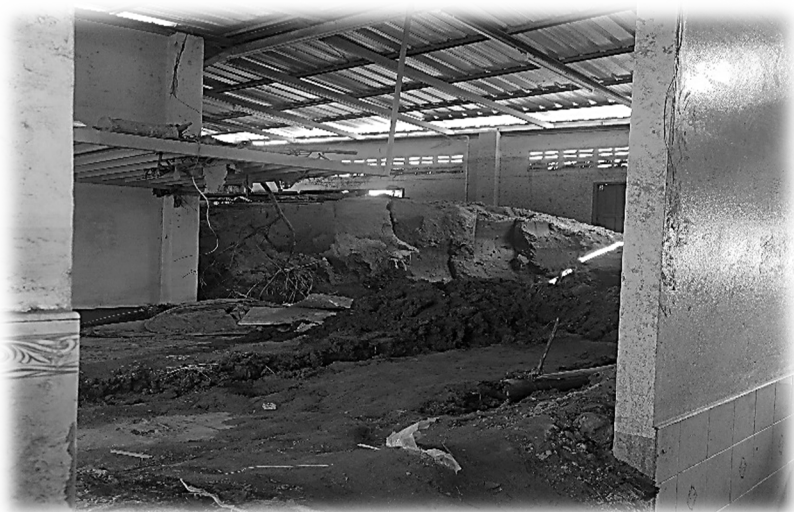
Photo 4: Damage from mud carried by floodwater, which has accumulated inside the houses of respondents in Mae Sai community. (Photo from the research site)
