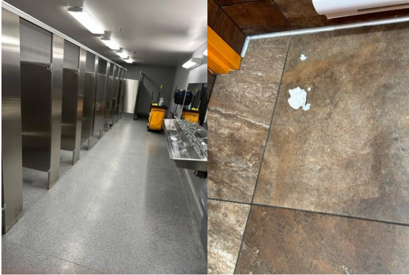
Figure 5.2a: Women's Public Restroom in Costco, Oshawa, Ontario (Source: Author, 03/5/23).
