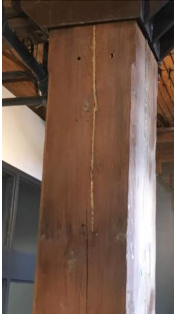
Figure 4.1. Partial attempted sealant repair on a radial crack present on a column.
