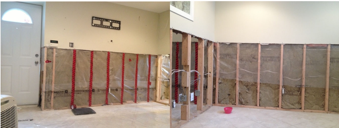
Lacaria, 2013: Recovering after the flood.
