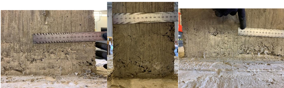
Figure 4.2: Locations of Poor Consolidation at the Toe Opposite the Actuator Side
