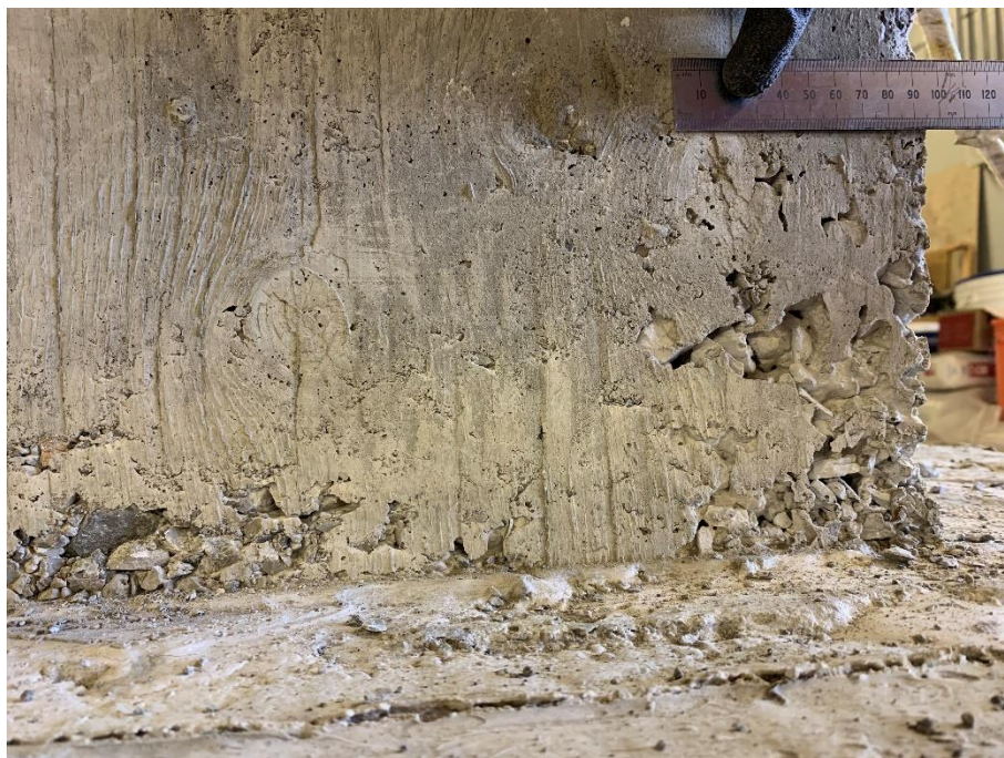
Figure 8.18: Honeycombing Along Base, Front of Wall, Non-Actuator Side
