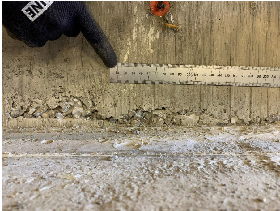
Figure 8.17: Honeycombing Along Base, Front of Wall, Actuator Side
