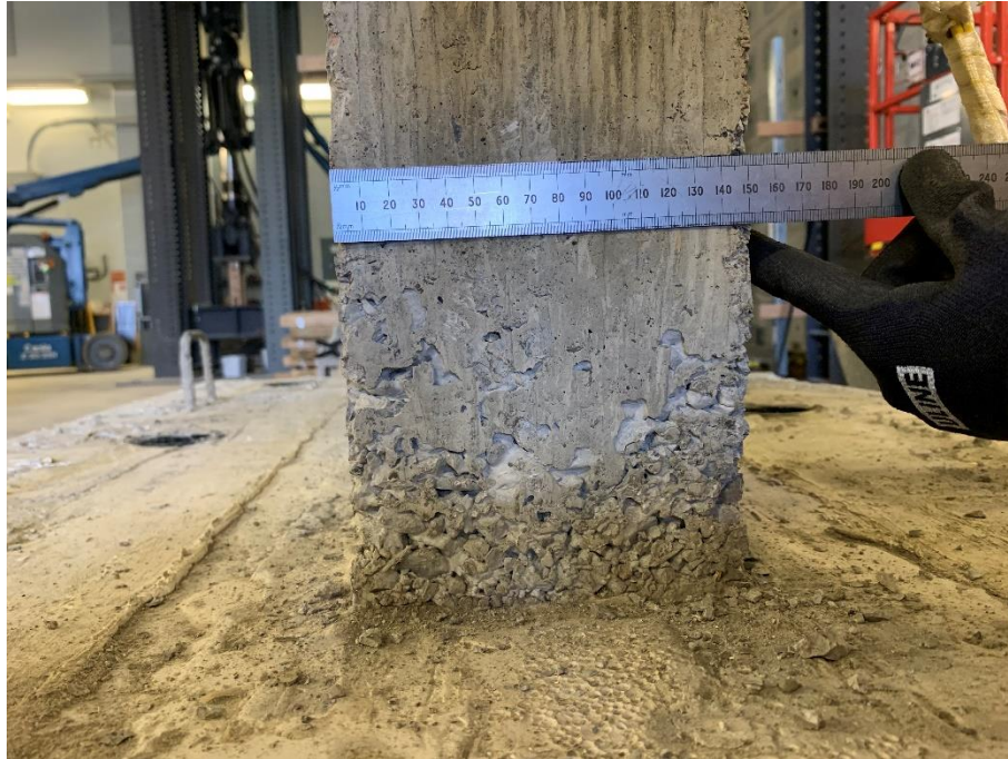
Figure 8.19: Honeycombing on Side of Wall, Non-Actuator Side
