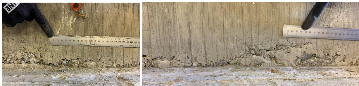
Figure 4.3: Locations of Poor Consolidation along the Base of the Front Face of the Wall
