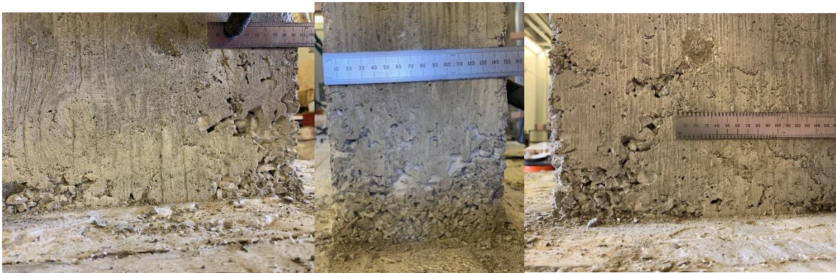
Figure 4.1: Locations of Poor Consolidation at the Toe on the Actuator Side
