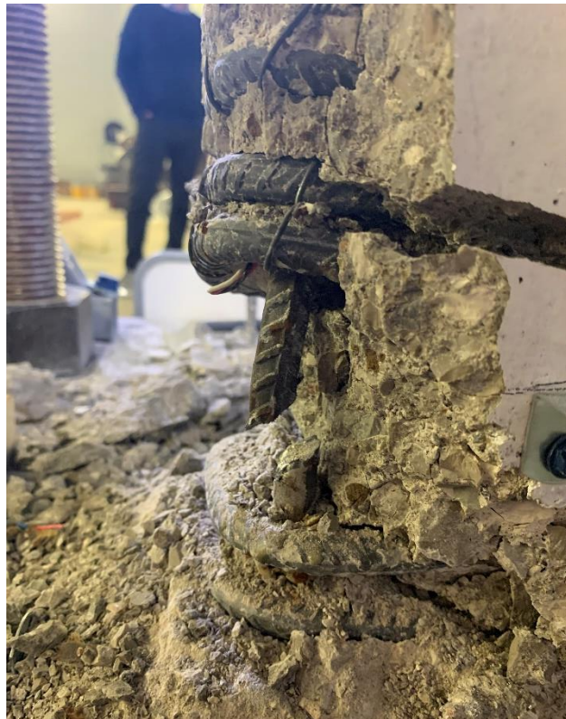
Figure 8.121: Rupture of Reinforcement in Boundary Region
