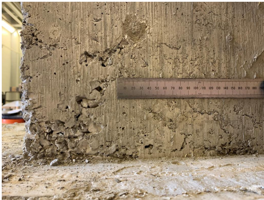
Figure 8.20: Honeycombing Along Base, Back of Wall, Non-Actuator Side
