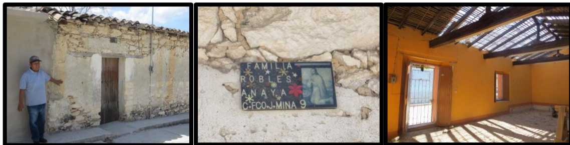
(a) Childhood home (b) Childhood home, detail (c) home at end of life
