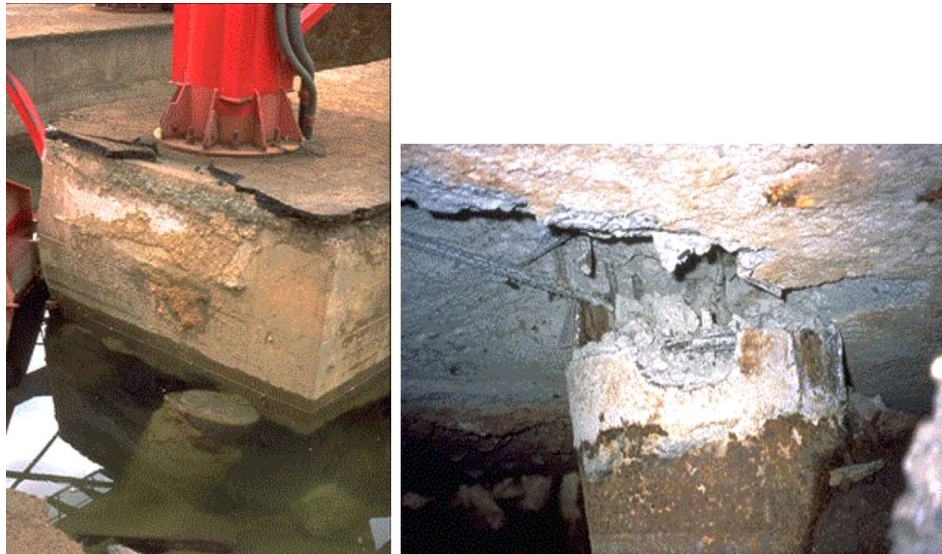
Figure 2-1 - Failure of pile to pilecap connection due to earthquake imposed load and soil pile interaction (Wei et al. 2008)
