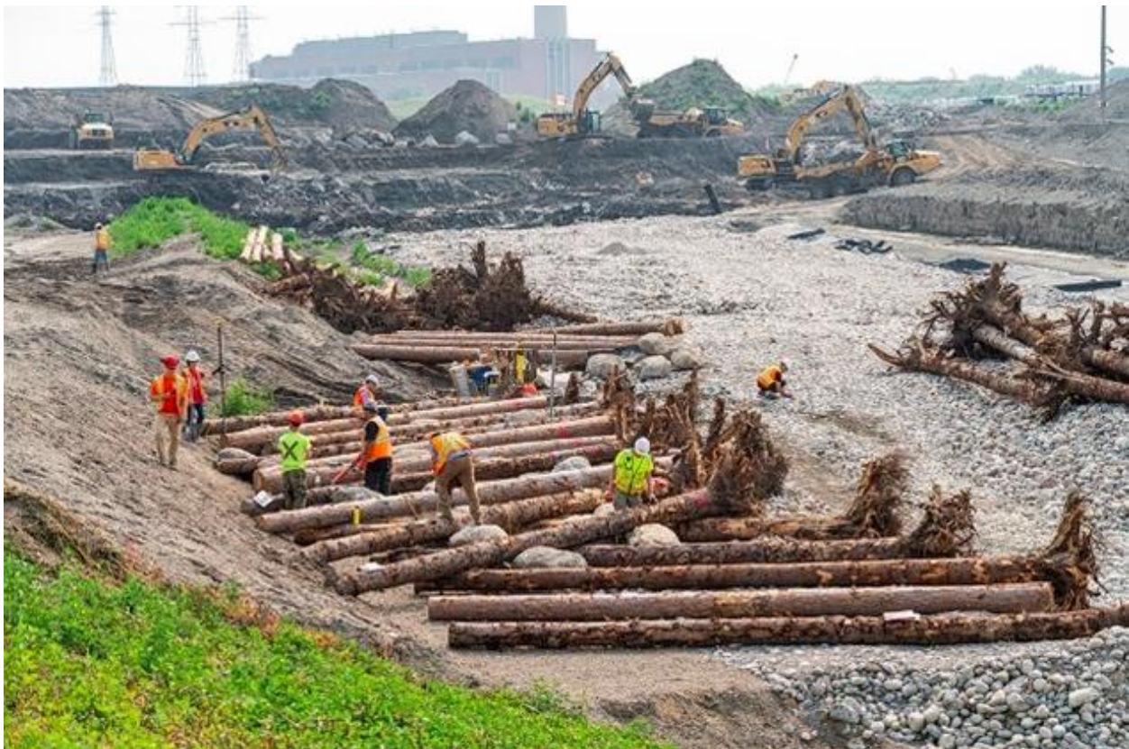
Figure 7. A photo of construction crew members setting tree trunks and root balls into new Don River shore. Image courtesy of Waterfront Toronto.
