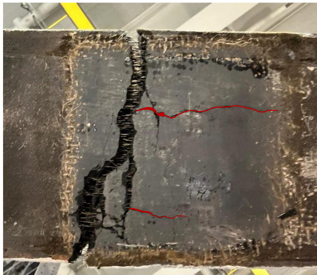
Figure 4-18. Bond Splitting of Bottom Cover of B4R1.5-1
