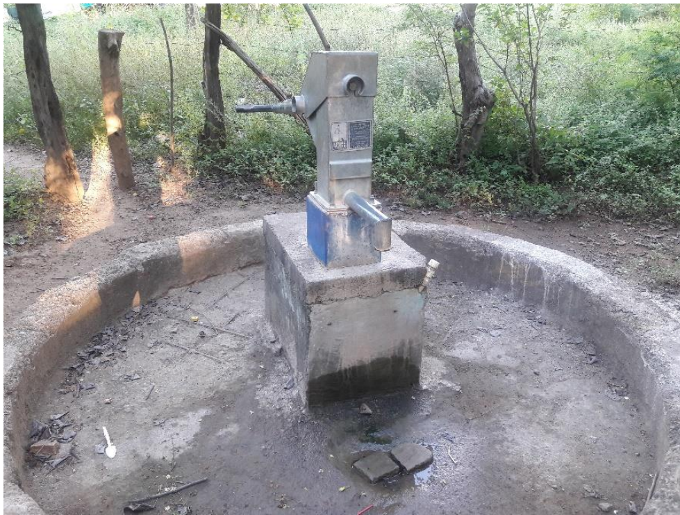
Hand pumped community water well in Las Mariitas.
