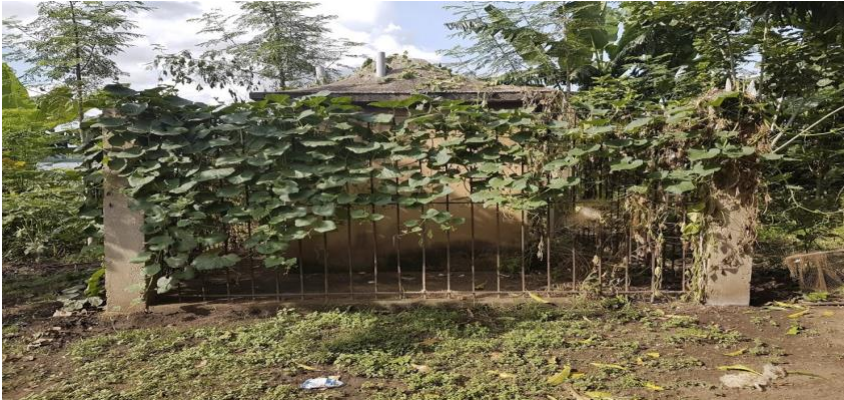
Figure 33 Early warning equipment, overgrown with weed and debris in Wurukum
