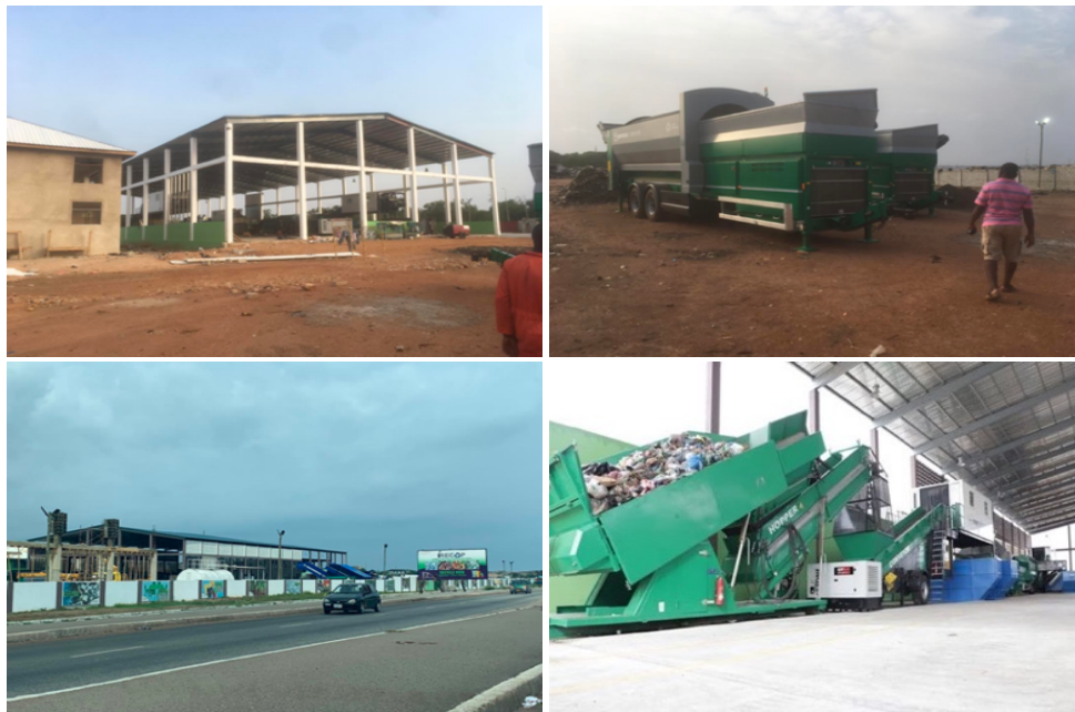
Photo 4. Construction of the new multifaceted waste recycling facility in Agbogbloshie. Source: Field assistant
